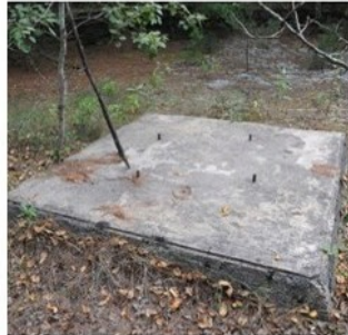
Remnant of the turntable at Howland Junction, the starting point of the IB&O railway.
